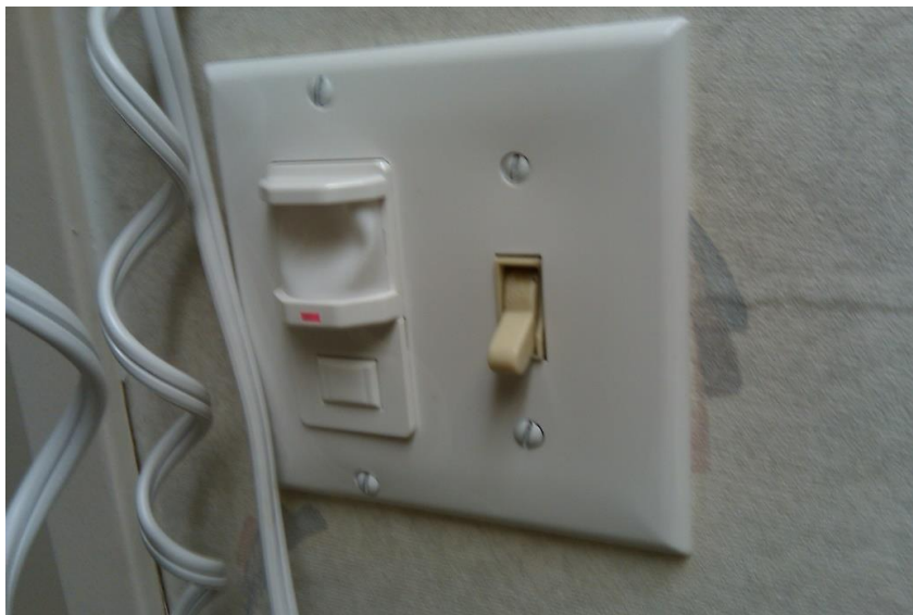
Figure 4-3: Wall Switch Integrated Occupancy Sensor Failure: Lens mistaken as button
